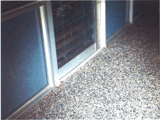
Figure 2.34 L1 base of south door
