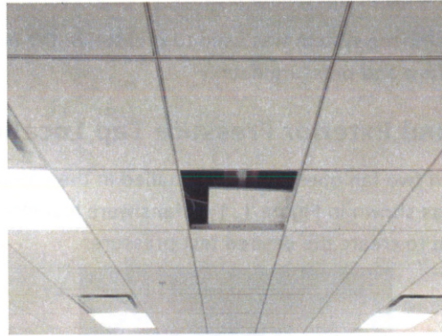
Figure 3 Ceiling tiles were removed during testing to create a single pressure boundary including the volume of the drop ceiling.
