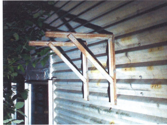
Figure 2.13 L1 exterior mounting bracket located on the Southwest corner
