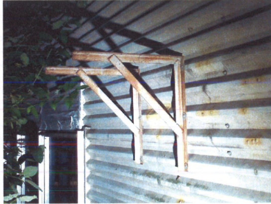
Figure 2 L1 exterior mounting bracket located on the Southwest corner
