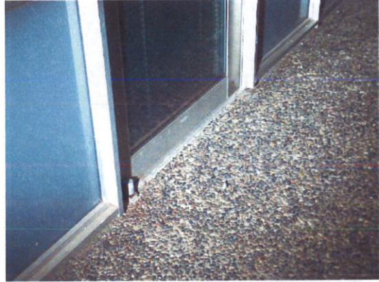
Figure 2.31 L1 southeast base of door
