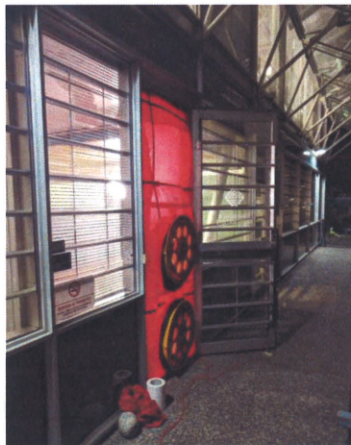
Figure 1 Blower door installed and sealed to the front door frame during pressurization testing.
