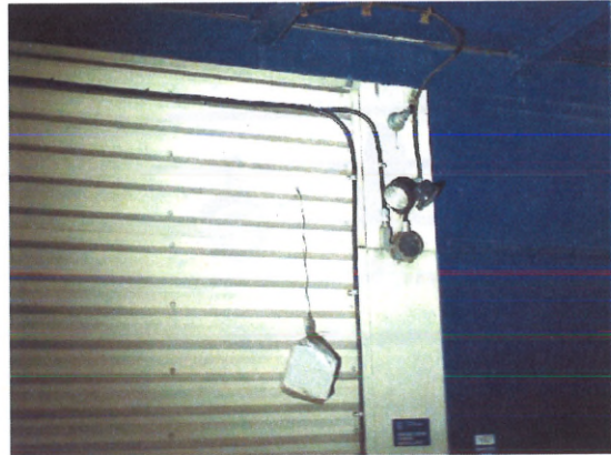
Figure 2.19 Hanging wire penetrations at the southwest corner
