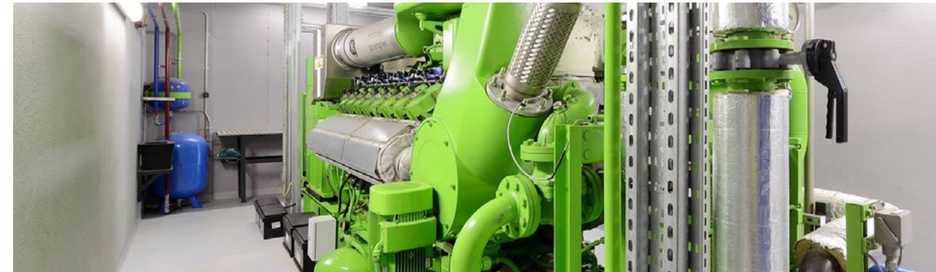
Combined heat and power (CHP) equipment, also known as co-generation equipment, produce electricity and heat that may be harnessed to provide heating and cooling to buildings. Clean burning fossil fuels like natural gas or propane are the typical energy sources for CHP plants that also provide as back-up power.
