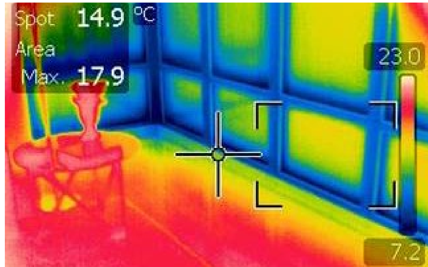
Thermography reveals thermal bridging in building enclosures causing discomfort at the outer perimeter of floor-to-ceiling glazing. Recent research has indicated that shelf angles, girts and fasteners can reduce the effective thermal resistance of walls by 50% or more. Inefficient windows cause occupant discomfort during very cold and hot weather.
