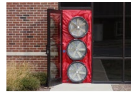
Airtightness testing during and following construction ensures a continuous air barrier system.
