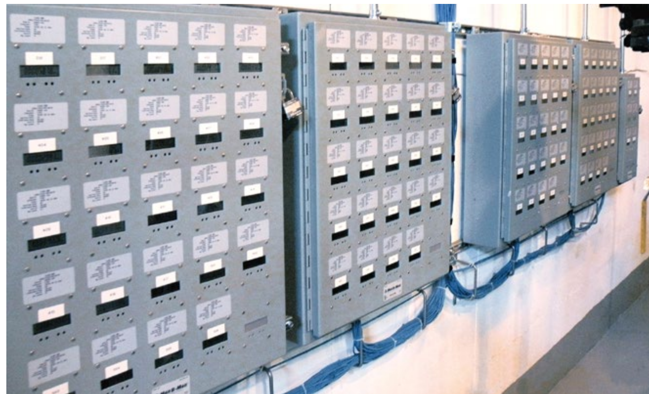
Digital submetering of electricity delivered to each suite in a MURB is now conventional technology. Advances in microprocessors and sensors have extended submetering to the flow of gases and fluids such that the use of centralized resources, such as domestic hot water or chilled water, can be accounted for at the individual suite level.
