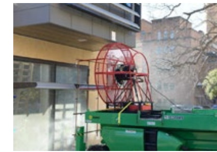
Field testing of windows and wall interfaces for moisture penetration avoids water damage and mold.
