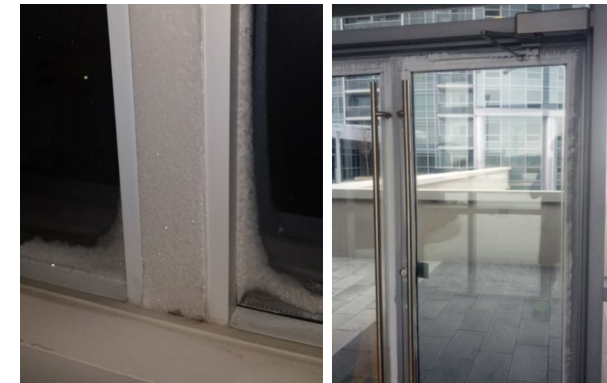
Frost and condensation build-up on the mullion of a window (left) and around the frame of a glass door (right). Moisture from the interior condenses on surfaces that are so cold due to thermal bridging that frost accumulates. Mold has started growing at the bottom of the window mullion and water will damage the window sill.
